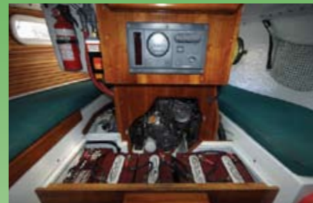
The Yanmar 1GM10C engine neatly installed in Velella
